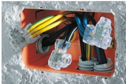
Examples of use of Z6-1, Z10-1 and Z16-1 terminals in junction boxes
